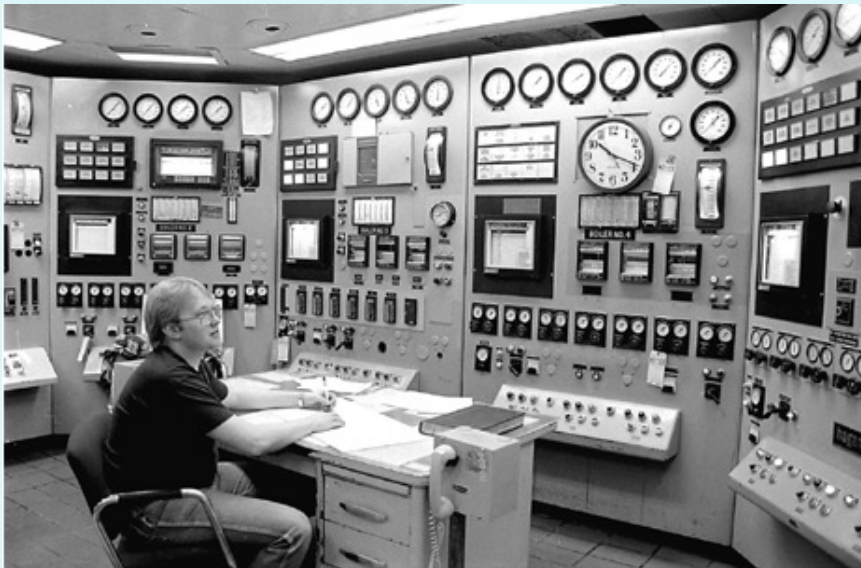
Boiler Operator Jeff Craigie sits in the Boiler Room and monitors flows, temperatures and pressures of the boilers and feed-water system. Photo by Ryan Solomon
