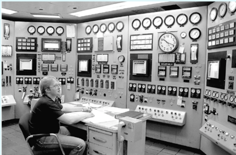
Boiler Operator Jeff Craigie sits in the Boiler Room and monitors flows, temperatures and pressures of the boilers and feed-water system. Photo by Ryan Solomon
